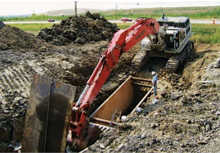
T+C employees make a deep sewer tie-in at a commercial business park site. The foreman standing on the bank is responsible for entering all daily data about the project into HCSS HeavyJob project management software.
