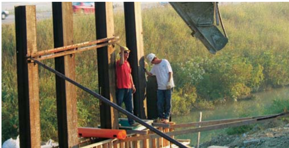
At a business park site, T+C employees pour concrete for abutment walls. All of their labor hours are recorded in HeavyJob software to maintain accurate records.
